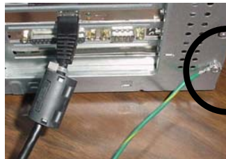
Ground Line on PC Chassis
