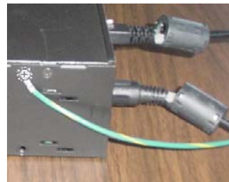
This partial view of a data acquisition device shows its connection to the ground-line. It also shows two ferrite collars, the foremost of which is clamped to the power cable. The background collar is clamped onto the Ethernet cable.
